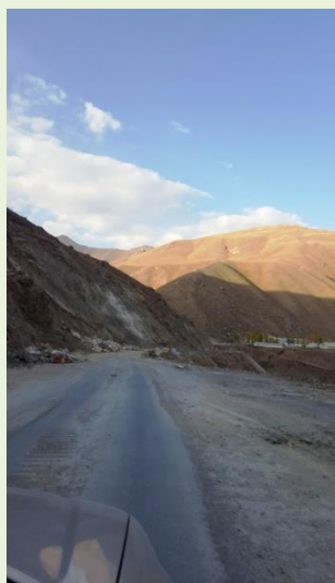
Poor road before the checkpoint «Jirgetal»
