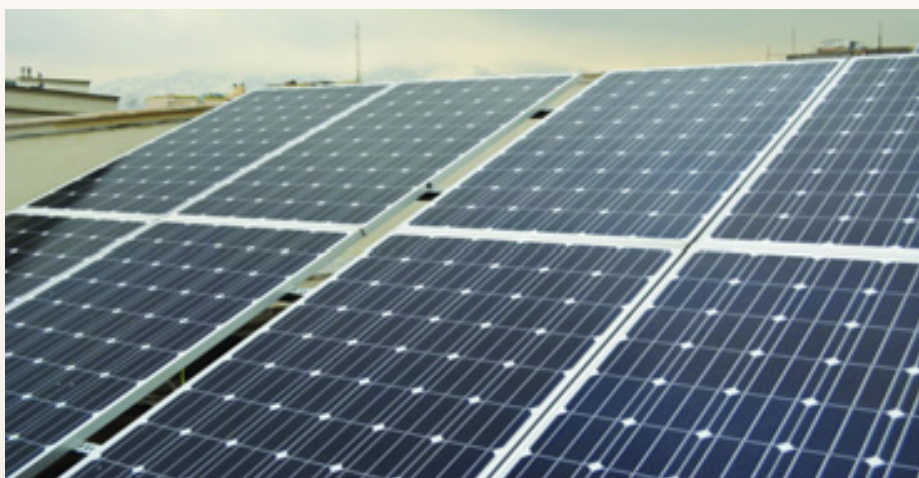
On-grid solar power plant on the roof of the ECO Secretariat
